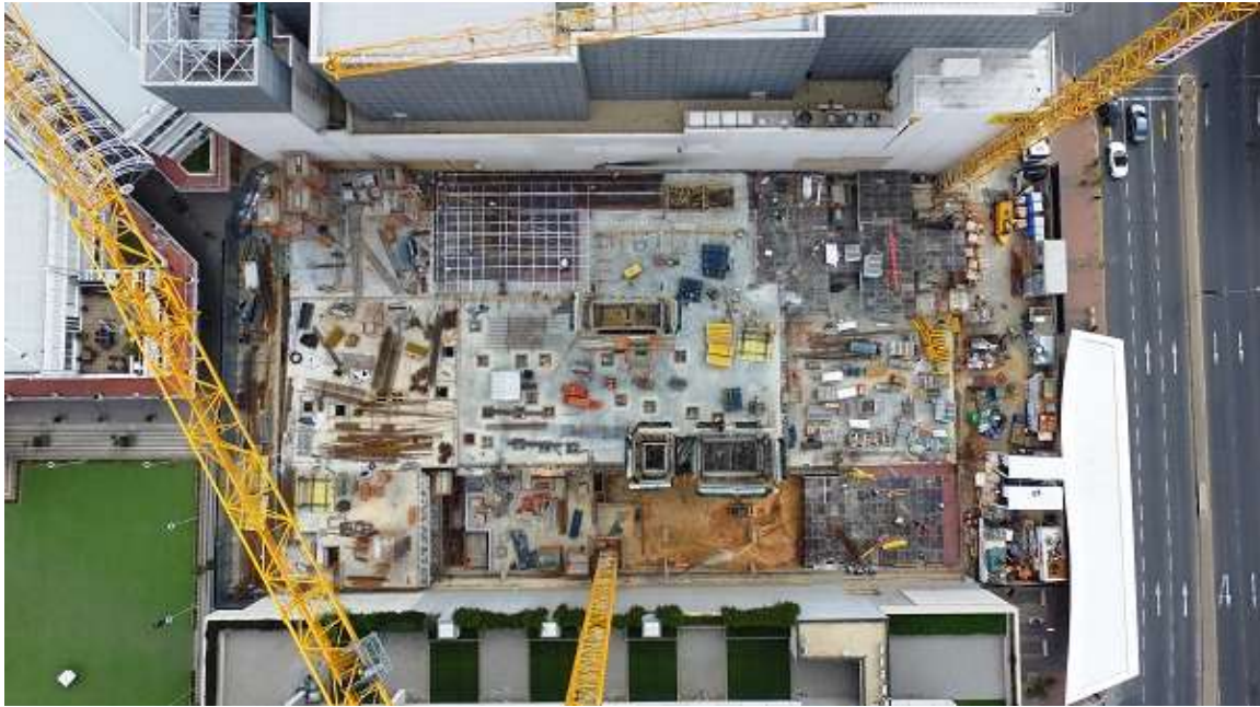
An aerial view of construction in the early days of the Rosebank Link. Credit: Paragon
