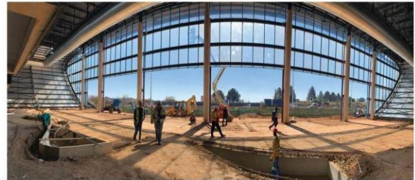
The challenges with the glass frontage revolved around securing the junctions of steel and glass, where straight meets curved - and ensuring weatherproofing of these joints
