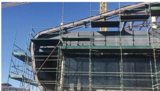
Large spanning trusses that carry a simplified roof were incorporated, sitting on a grid that can accommodate the different sized equipment sizes equipment
